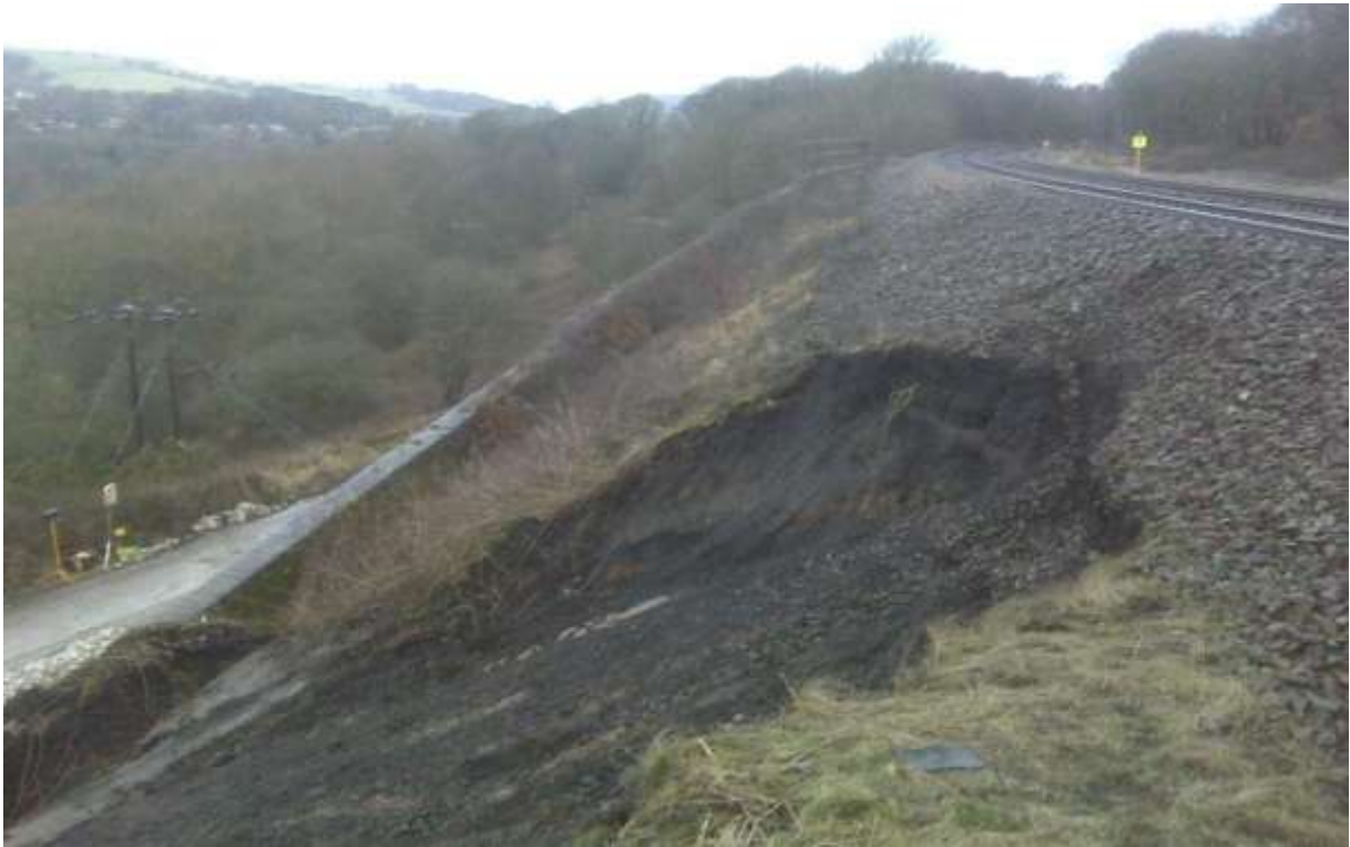
Fig. 1 Landslip at Bugsworth, 7 February 2011. (Courtesy NetworkRail)
